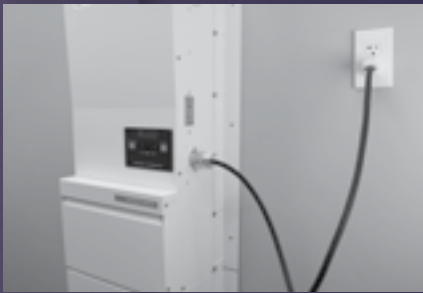
BATTERY BACKUP SYSTEM
